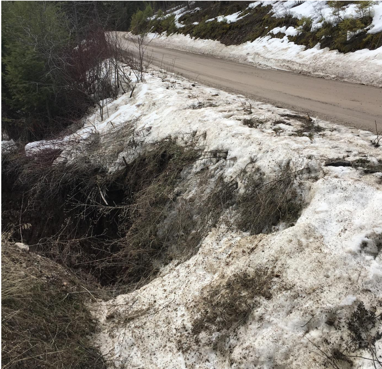
Photo of Landslide Zone #5, March 15, 2017. The landslide has occupied essentially the same failure location as before.
