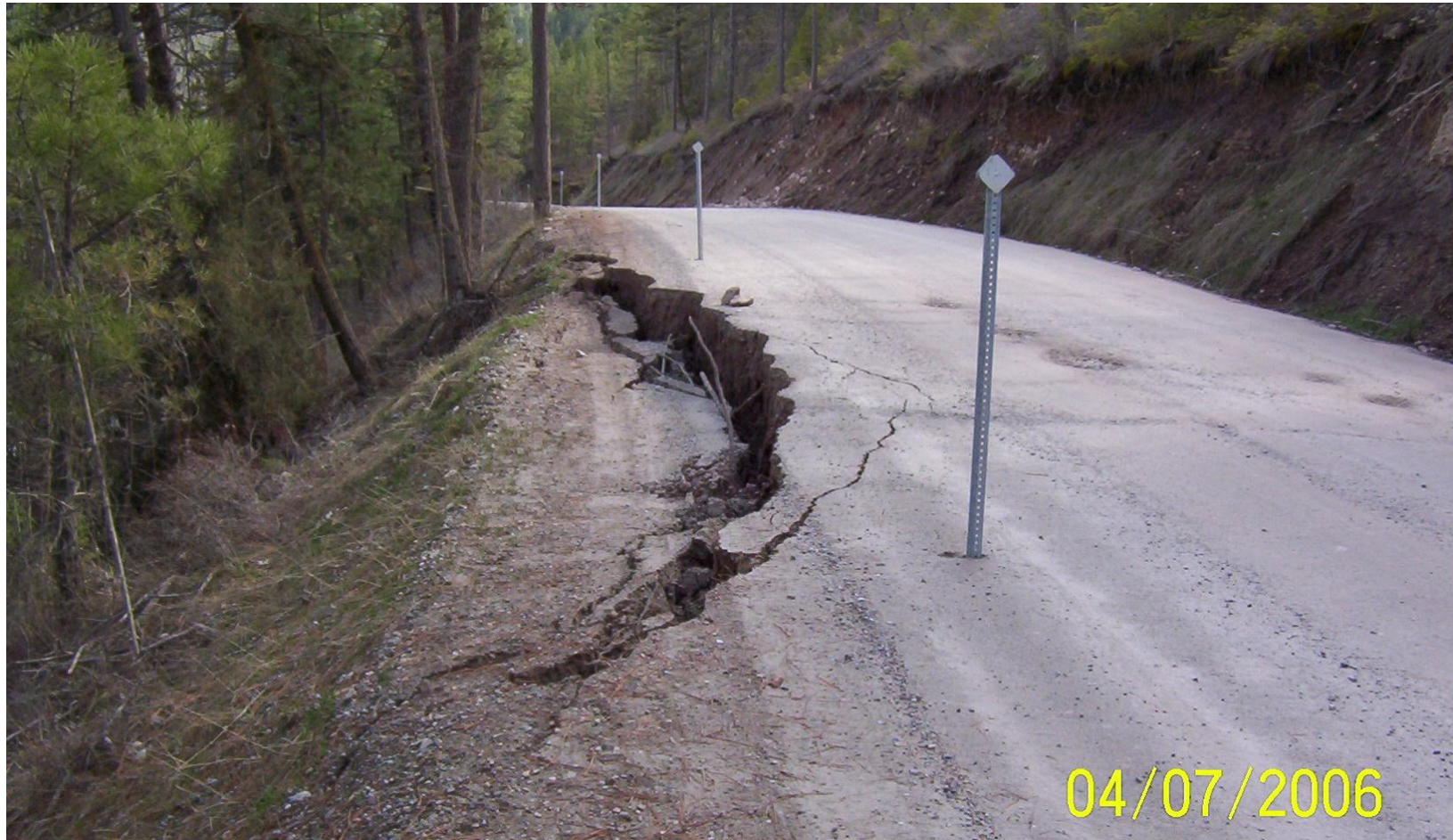
April 7, 2006 Photo of Landslide Zone #1. The upper edge of the scarp extends approximately 8 feet into the road from the crest of the slope. At this time, the scarp extends about 45 feet along the slope crest. This slide was repaired but would continue to periodically fail, including a March 2017 failure (see Exhibit A-4)
