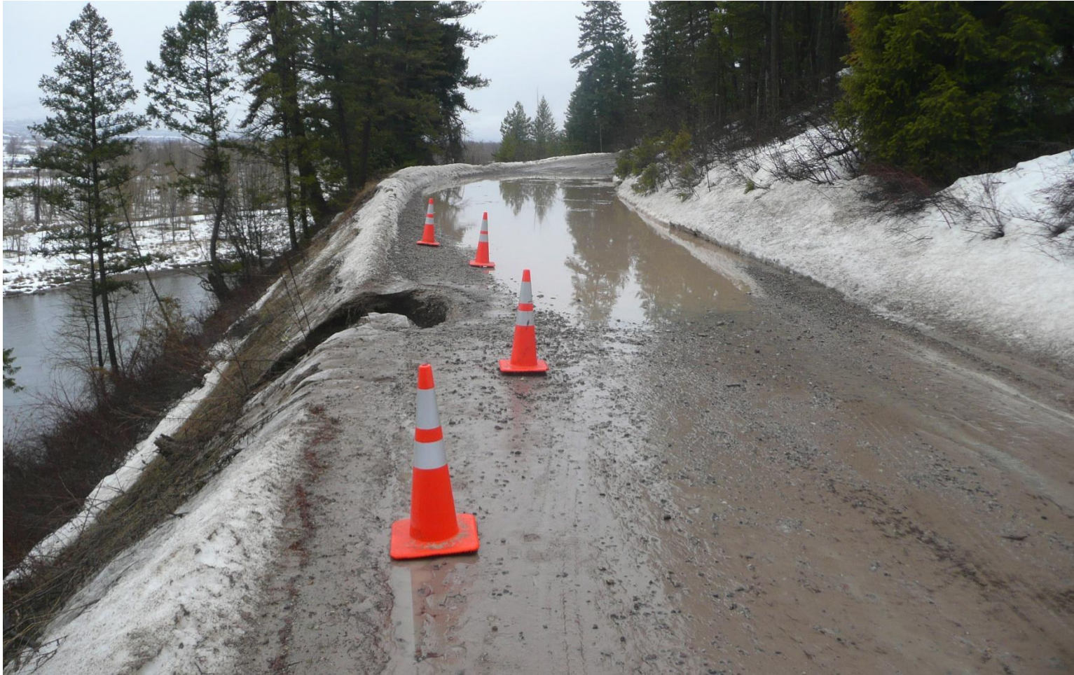
This photo, taken March 10, 2014, shows both an erosional event (due to poor roadway drainage) as well as small-scale landsliding at Landslide Zone #6. Note the tilted trees in the background that are exhibiting various degrees of slope creep.
