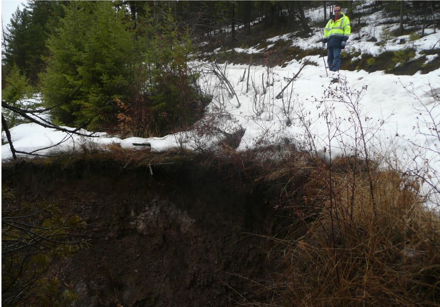
Landslide at Zone 5, March 10, 2014. This slide is located at the outside edge of the road. Note the relatively young trees that are tilting downhill in the immediate background of this scene, indicative of slope creep beyond the landslide limits.
