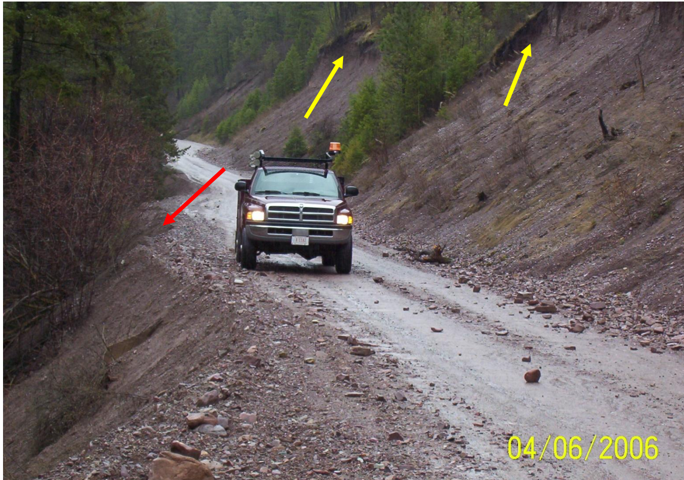
Photograph of landsliding and slope erosion along Landslide Zone #7. The yellow arrows above the road indicate uphill-propagating landsliding, the same as the large-scale landsliding observed in Landslide Zone #4 below the current Big Flat Road. The red arrow indicates the small-scale landsliding that is observed along much of this reach of Big Flat Road.
