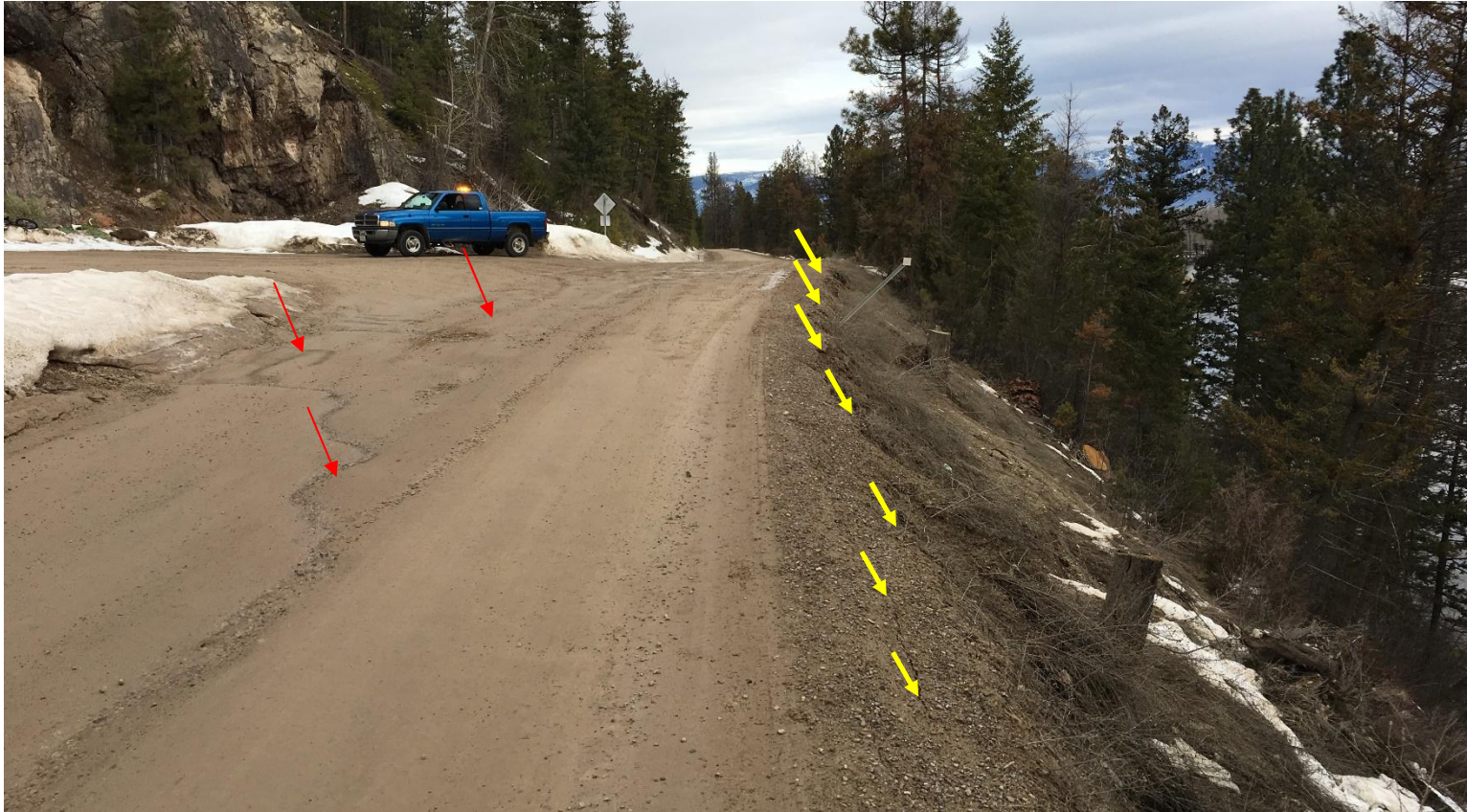
Photo of the Zone 2 Big Flat Road Landslide on March 13, 2017. The 2017 landslide crest is delineated by the yellow arrows, and an older scarp, not well developed but in the roadway, is shown by the red arrows. The 2017 slide did not develop to the extent of earlier slide episodes, but did undergo movement nonetheless.
